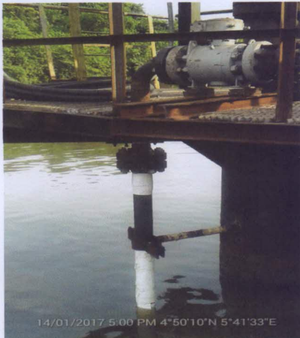
FIG 3: Spill point after repairs
