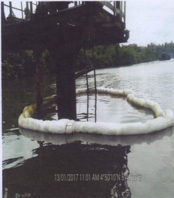
FIG: 1 Spill point on arrival at site
